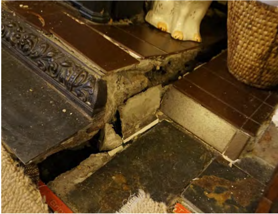
The heating pipework pulled apart
